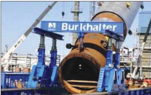
Figure 41. Hydraulic gantry and tower lift system.
